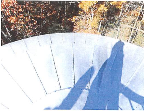
Roof exterior: showing coatings to be heavily chalked and moderately soiled in areas.
