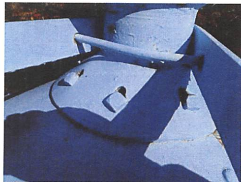
Roof exterior: showing open penetrations resulting from slotted bolting holes at the base of the finial ball.
