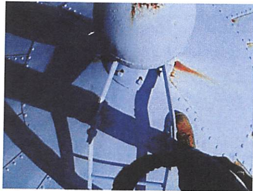
Roof exterior: showing rolling revolving ladder is securely attached to the finial ball.
