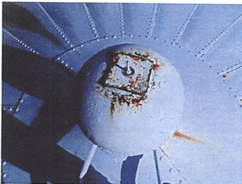
Roof exterior: showing scattered coating failure and rusting along top of finial ball and its rigging port.
