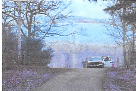
Workers have just started to rehabilitate the 50 years old Hill Street water tank.
