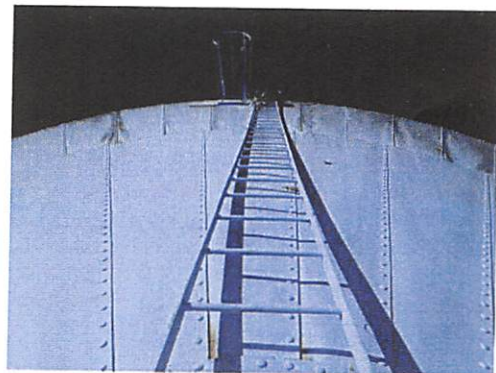
Roof exterior: showing revolving ladder to be intact and in good structural condition.
