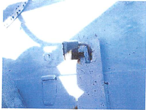
Roof exterior: showing hatch cover equipped with a locking hasp and lock which was secured in place prior to and after inspection.
