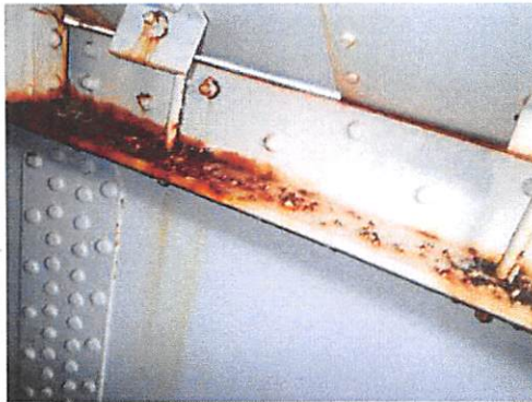
Roof to shell junction: showing extensive coating failure and heavy rusting along top face of rim angle and J-bolt assemblies.
