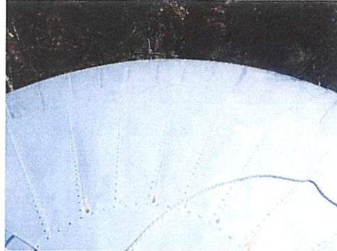
Roof exterior: showing coatings to be in fair to good condition with only minor degradation and localized rusting taking place.
