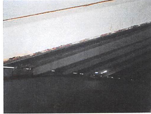
Roof to shell junction: showing slight gaps between shell wall and roof plates along entire perimeter
