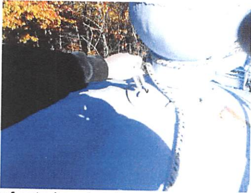
Roof exterior: showing open penetrations resulting from slotted bolting holes which appears to penetrate to inner surfaces.
